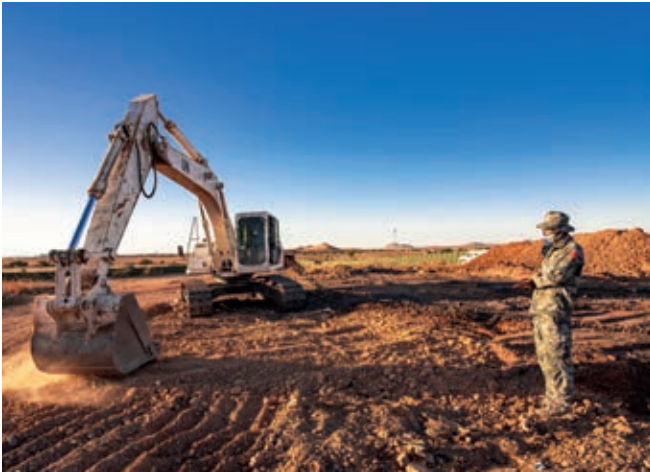
China's peacekeeping force repairs a road in Darfur Sudan on February 23. Xinhua
