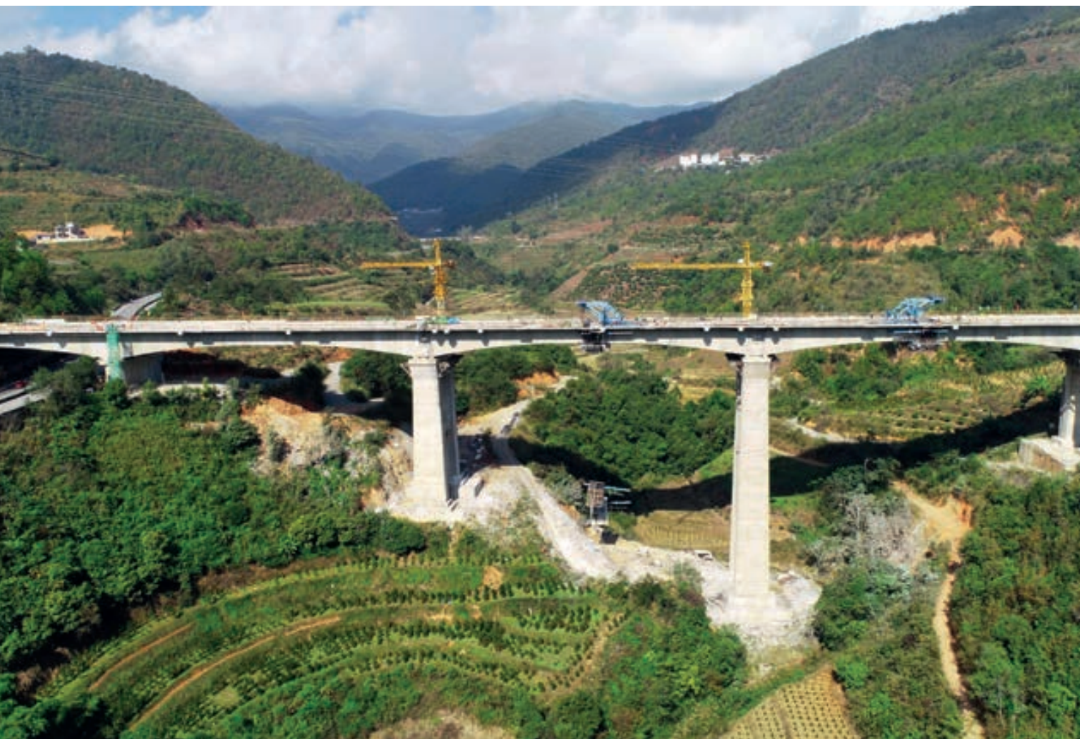
The Yuxi railway bridge in Southwest China's Yunnan Province, which is the first four-lane railway bridge of China-Laos Railway realizes closure on January 16. Chen Chang
