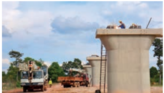
The construction site of a bridge along the China-Laos railway on May 2 in Vientiane, capital of Laos Liu Ailun
