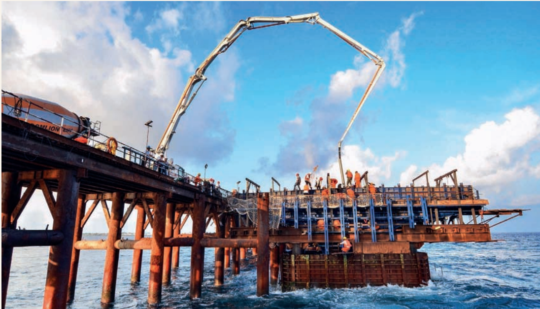
The photo taken on April 21 shows the construction site of the China-Maldives Friendship Bridge. The bridge, which connects Malé, capital of Maldives, to the airport island Hulhulé, serves a symbol of Sino-Maldivian friendship. Xinhua
