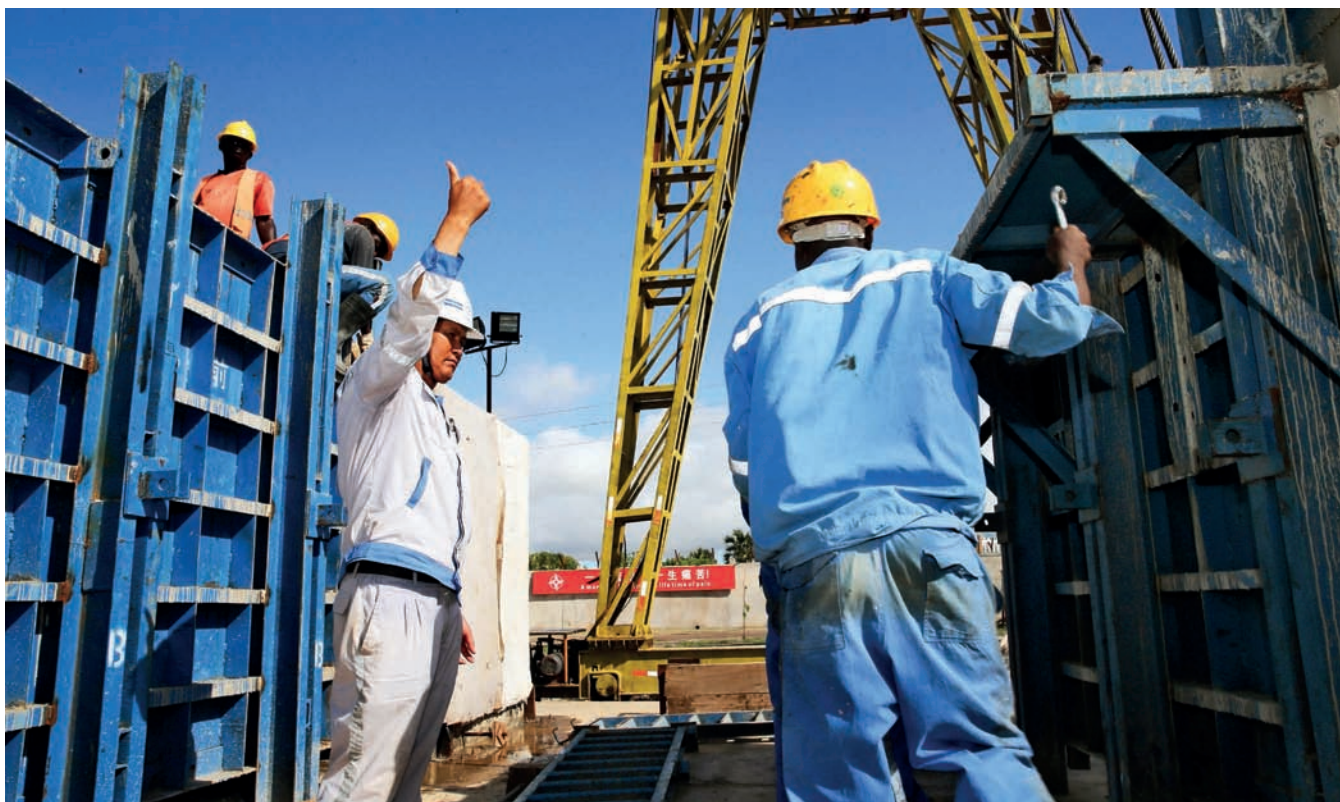
Liu Xingze (L, front), a Chinese technician, works with his Kenyan counterparts to upgrade the Lamu Port in northeastern Kenya on May 10. Pan Siwei
