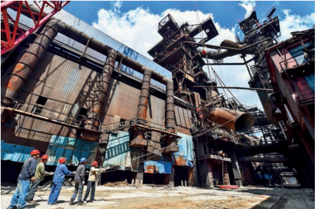
Workers from Baogang Group dismantle a steel-making stove in Baotou, Inner Mongolia Autonomous Region on August 31, 2016, which helped cut the production capacity of 1.33 million tons annually. Lian Zhen
