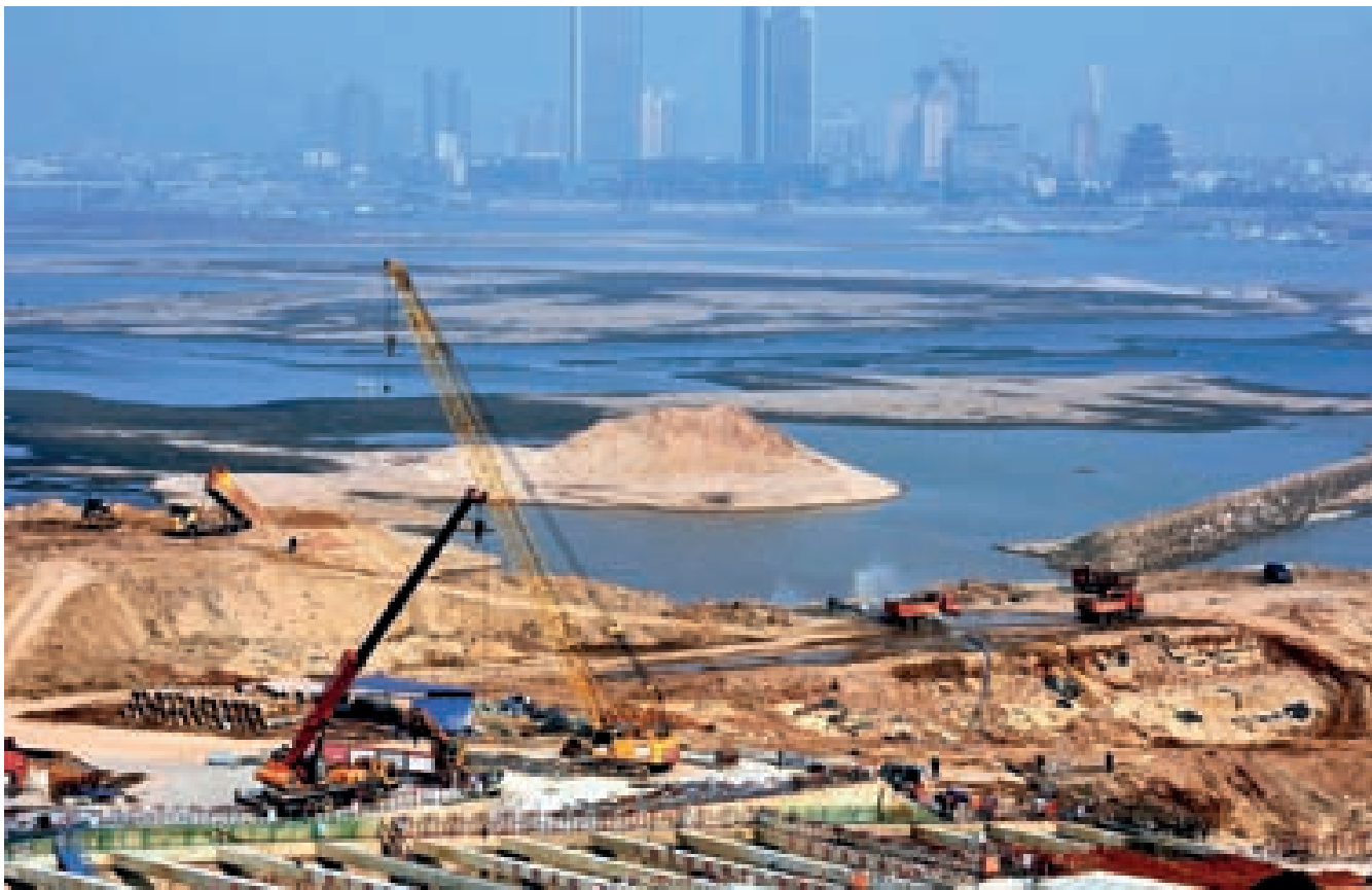
The construction site of a PPP (public-private partnership) project in Nanchang of Jiangxi Province on February 8 Song Zhenping
