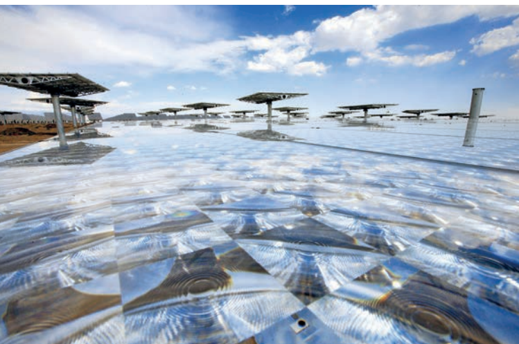
A photo taken on June 20, 2014 showing the photovoltaic power generation equipment concentrating solar is to be set up by Xinjiang Hami Ephi Solar Energy Ltd. Li Mingfang
