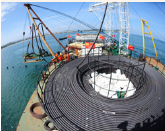
Workers with the Changdao Power Supply Company under the State Grid lay submarine cables on September 2, 2012. Chu Yang
