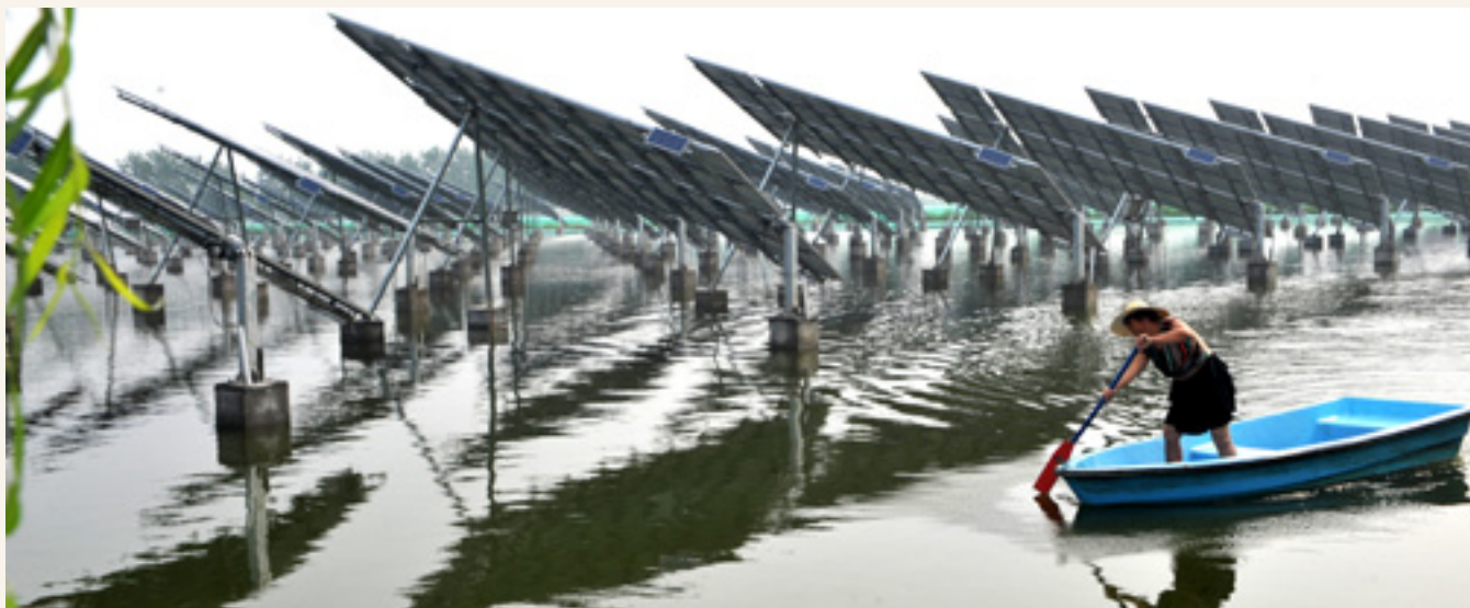
An employee works at a solar photovoltaic power station established in a fishpond on August 19, 2012 in Jianyang Township, Jianhu County, Jiangsu Province. It is the first photovoltaic power station built in the province, which conserves energy and reduces emissions by successfully combining aquaculture and power generation. Pu Liangping
