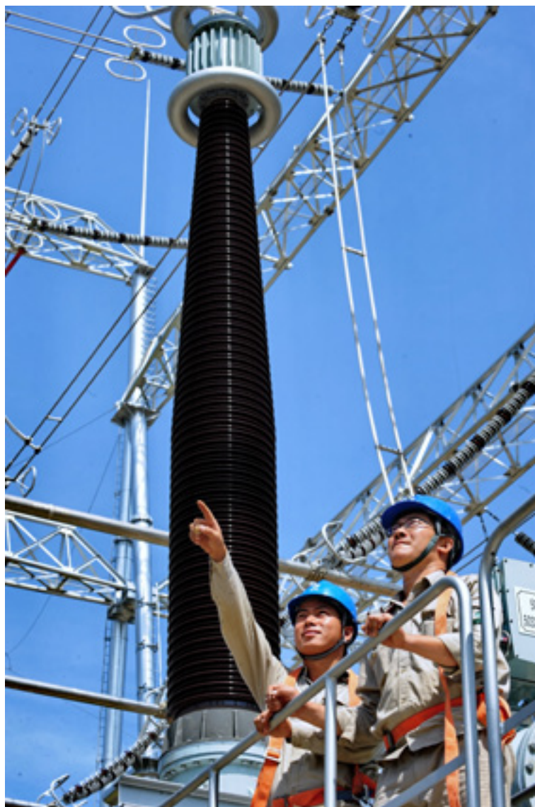
Two workers with the Fujian branch, State Grid Corporation examine power transmission equipment at the Lili Converting Station on September 28. It is the first 500-kilovolt intelligence converting station installed in Fuzhou, capital of Fujian Province. Zhang Guojun
