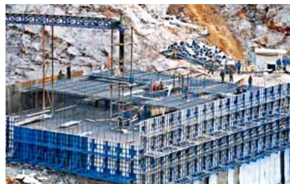
Builders from Sinohydro Corporation work at the construction site of middle route of the South-North Water Diversion Project. Xinhua
