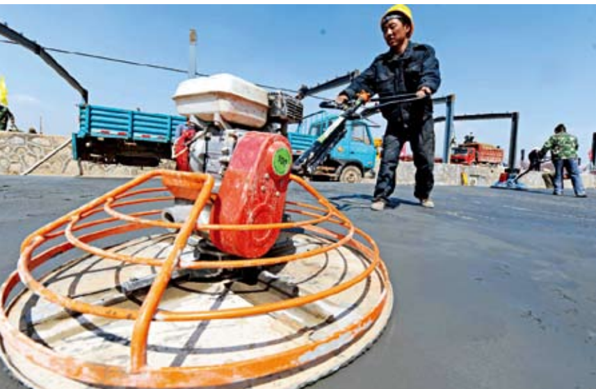
Employees of the China Railway 21st Bureau grind the road of the earthquake rescue and relief center at the Xining North Cargo Transportation Station in Qinghai Province. Hou Deqiang
